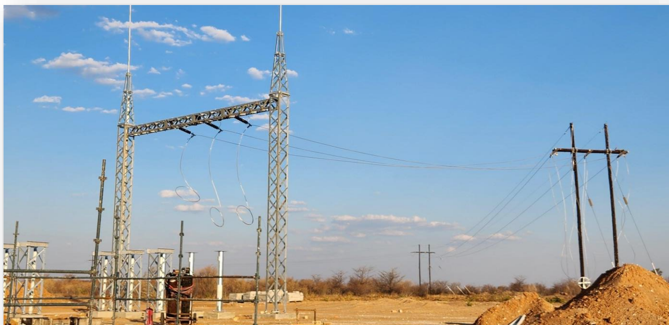
Lesedi Substation and Transmission Line connection
